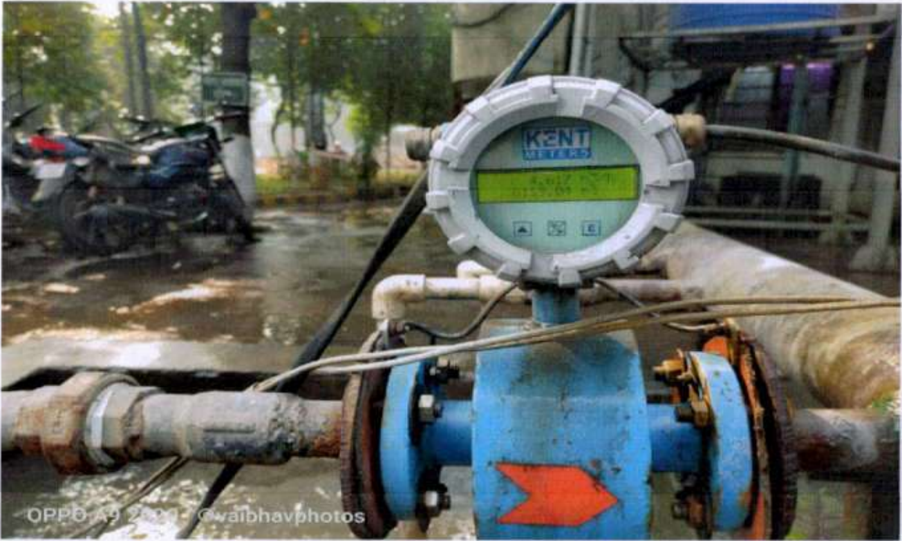
Digital Water Meter in Bore at Gate No. 3
